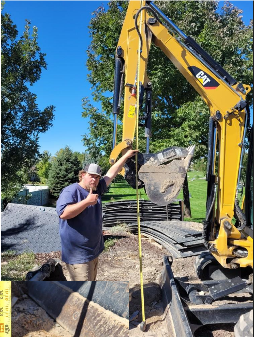
New Building Doors need to be able to accommodate 12' 5" equipment height
